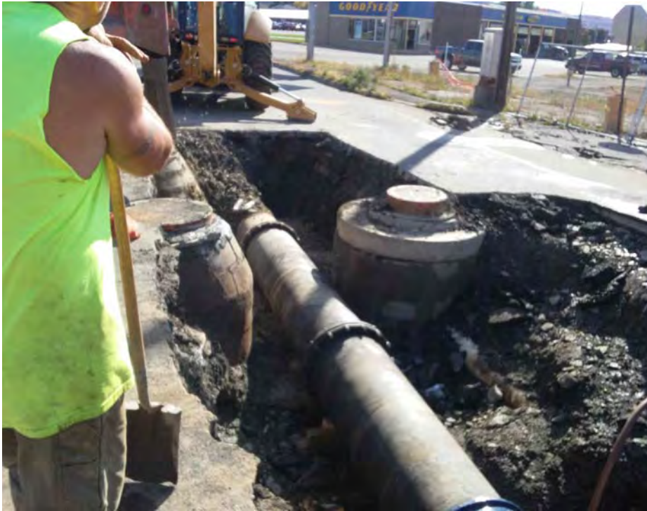
Harrison Ave 24" Water Main
